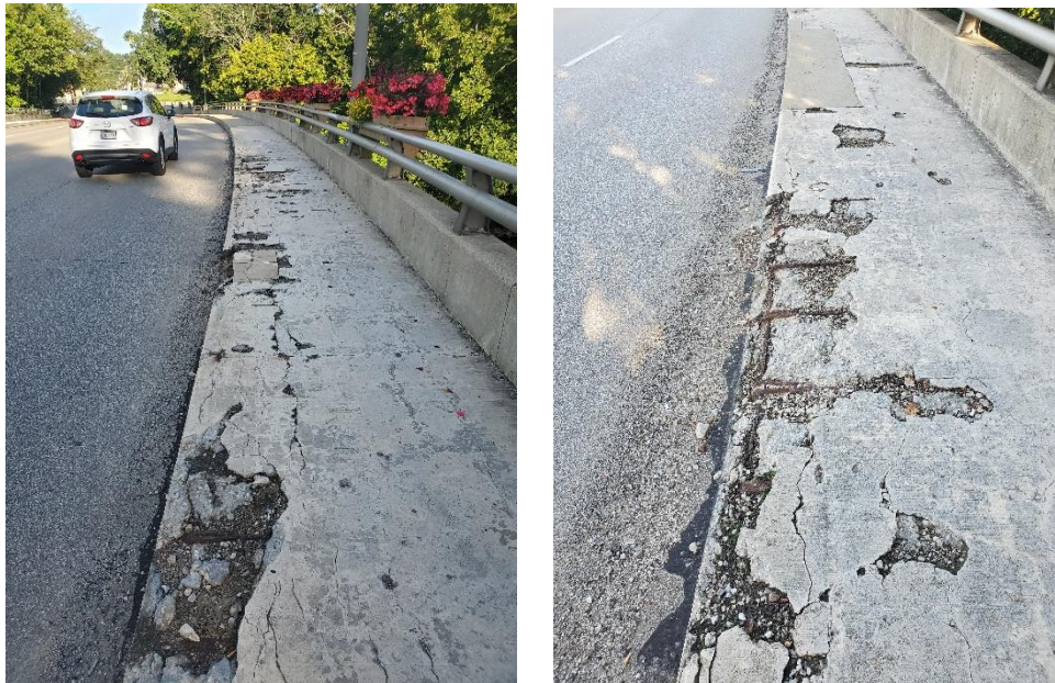
West Loveland Bridge Sidewalk Conditions
