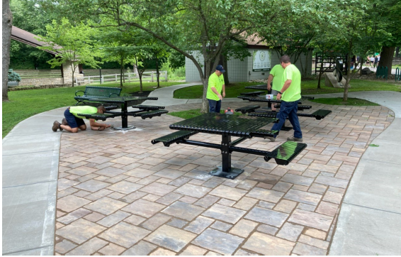
Improvements to Nisbet Park continue as Public Works installs tables in the new seating area
