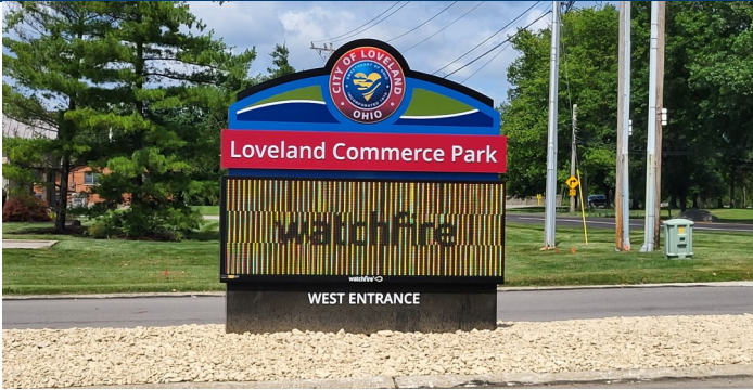
New Message Center Sign installed at the entrance to the Loveland Commerce Park
